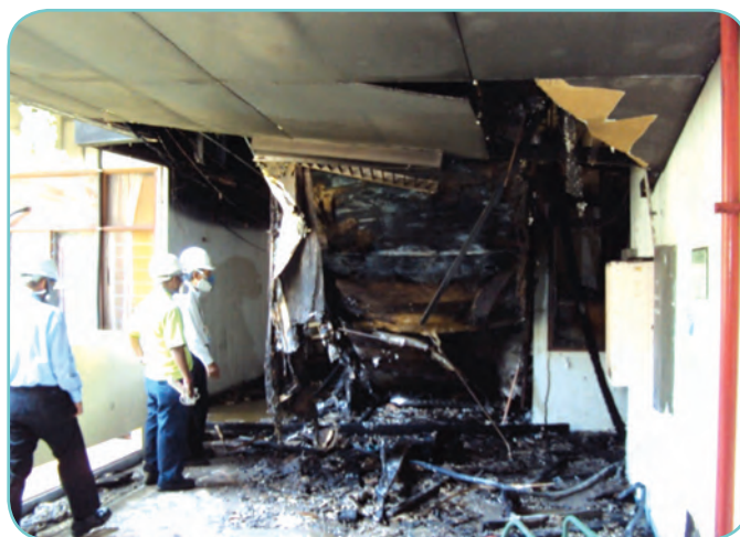
IMAGE 12 AFTERMATH OF FIRE AT IMR, 18 APRIL 2011
